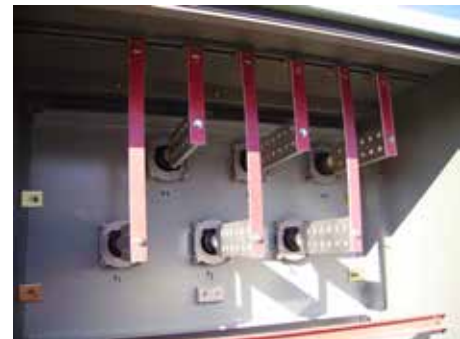
Figure 11. 12-pulse application with bushing supports.
